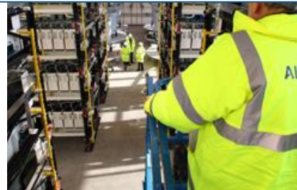
Alstom Grid UK HVDC Power Systems
