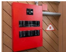
Fire control panel and safety systems
