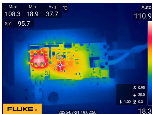
Figure 3-79. Bottom Side at 90Vac-to-20V/3.25A
