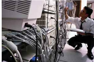
Heavy Traffic Over Ethernet
